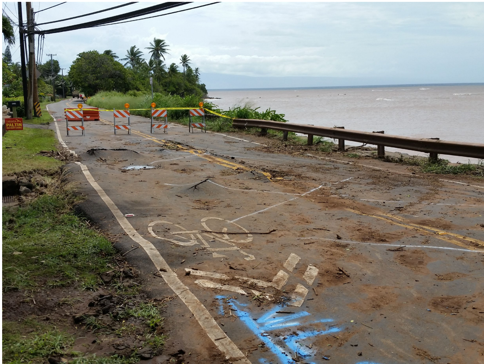
Figure 11. Damage to Kahaha Road in Napili area (Credit: Maui Emergency Management Agency).
