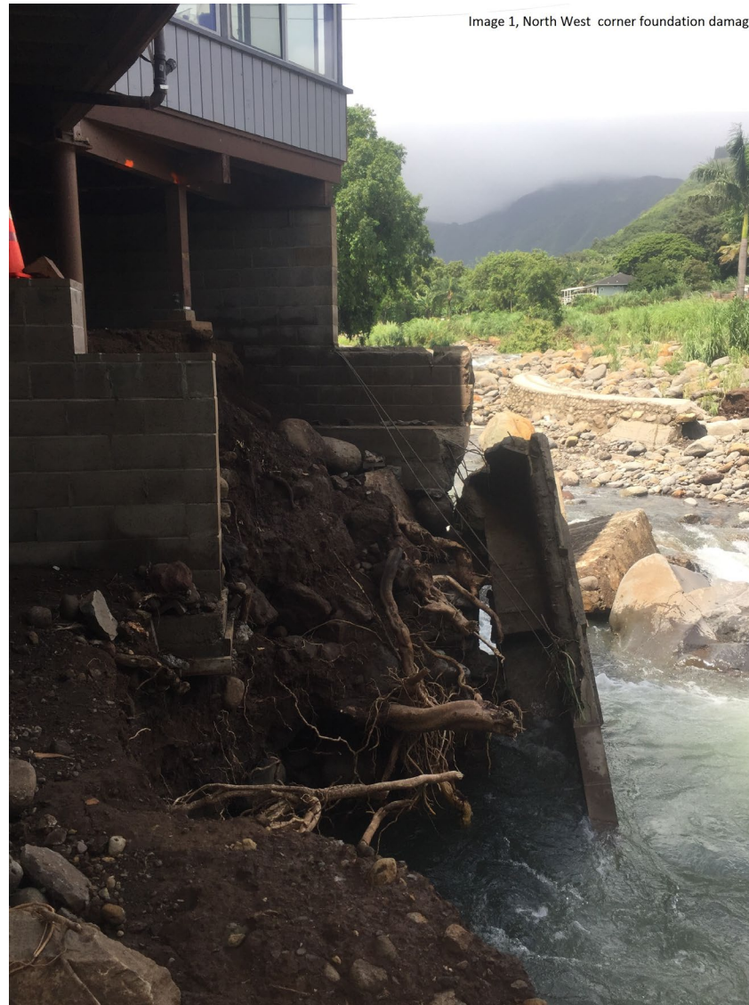
Figure 12. Home in Waihee River Basin with foundation damage (Credit: Maui Emergency Management Agency).
