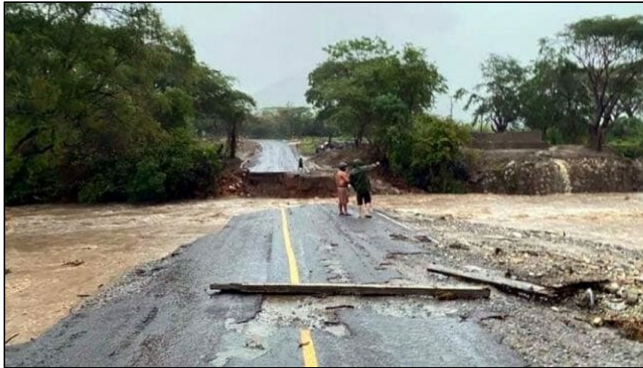
Figure 6. Collapsed bridge in Colima. Image courtesy of Mexico News Daily .
