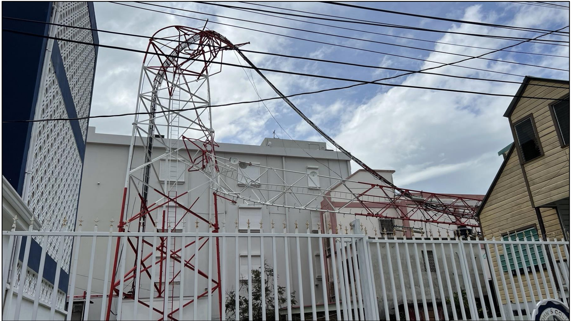
Figure 6. A downed metal communication tower in downtown Belize City. Image courtesy of Josh Morgerman (iCyclone).
